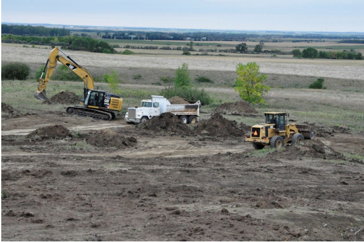
Figure 11: Sinkhole filling at the Quist Site.
